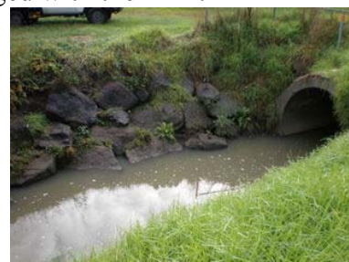
Figure 9: Lillimur Stormwater Drain
